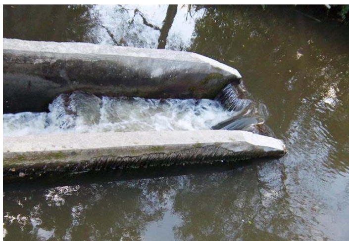
The alterations involved reshaping the leading edge of the pass to prevent debris building up and replacing the pipe with a notched weir to improve access for fish.
